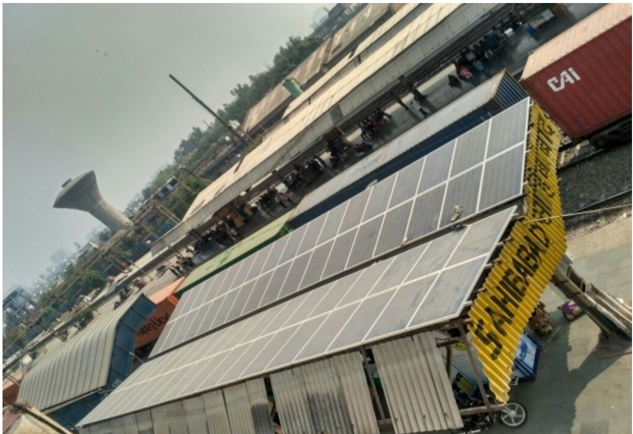
Solar Panel directly mounted on platform structure : first time on Indian Railways
